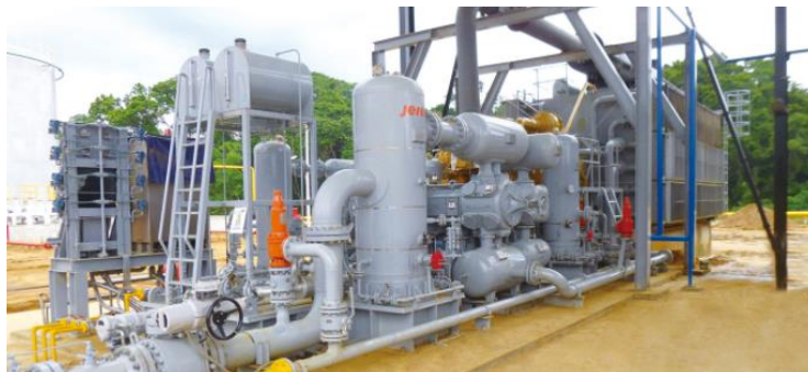
Figure 7: Gas compressor (Jereh Oil and Gas)
